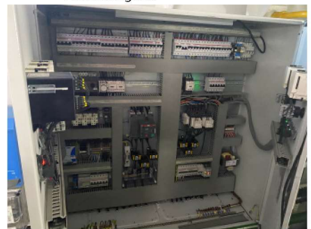
Electrical Control System
